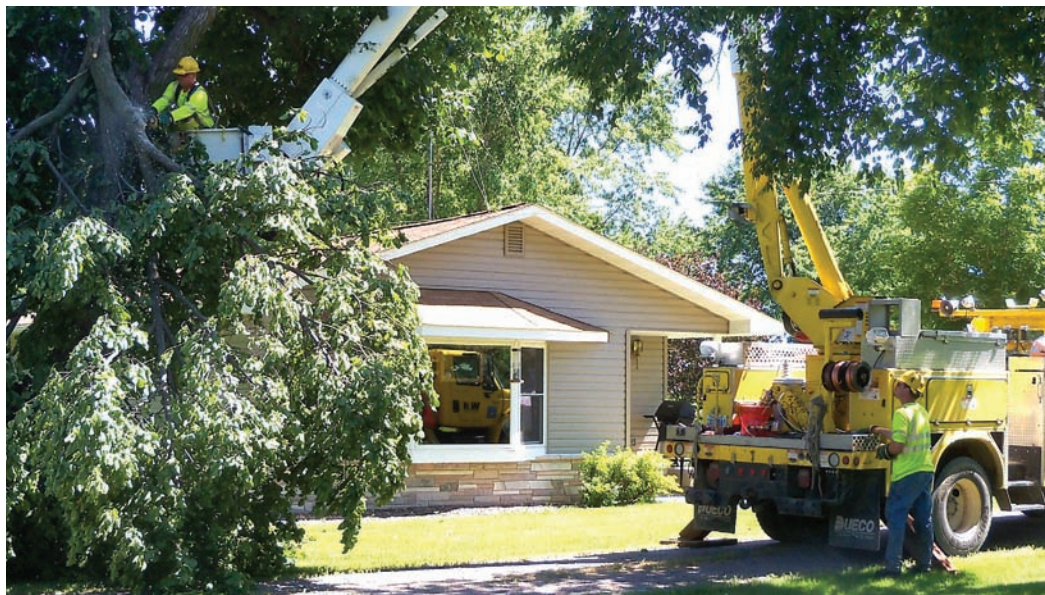
Line crews worked around the clock from July 1-3 to restore power. A number of downed trees slowed their progress.
